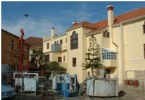
When building on sand, especially above an ancient rubbish tip, one must provide your own rock. In May this year, George Whitfield College, Capetown, commenced building its new study centre. The Study Centre will stand on 35 x 8 metre steel reinforced pillars cast in holes drilled into the ground. The Centre will house the library which includes books donated from various places in Australia.
